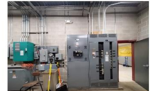
EXISTING ELECTRICAL GEAR
