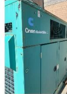
EXISTING NATURAL GAS GENERATOR
