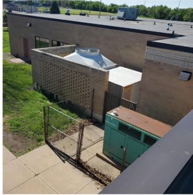
EXISTING COOLING TOWER, PUMP SHED, GENERATOR
