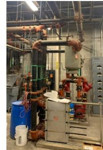
EXISTING STEAM TO HOT WATER HEX & CONDENSER WATER PUMPS
