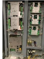
EXISTING AUTOMATIC LOGIC CONTROL PANEL
