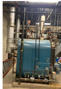
EXISTING STEAM BOILERS
