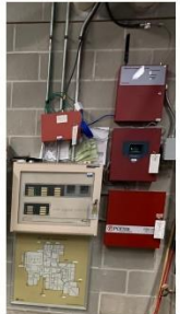
EXISTING FIRE ALARM SYSTEM PANELS
