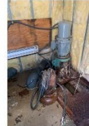
EXISTING COOLING TOWER PUMP
