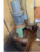
EXISTING COOLING TOWER PUMP
